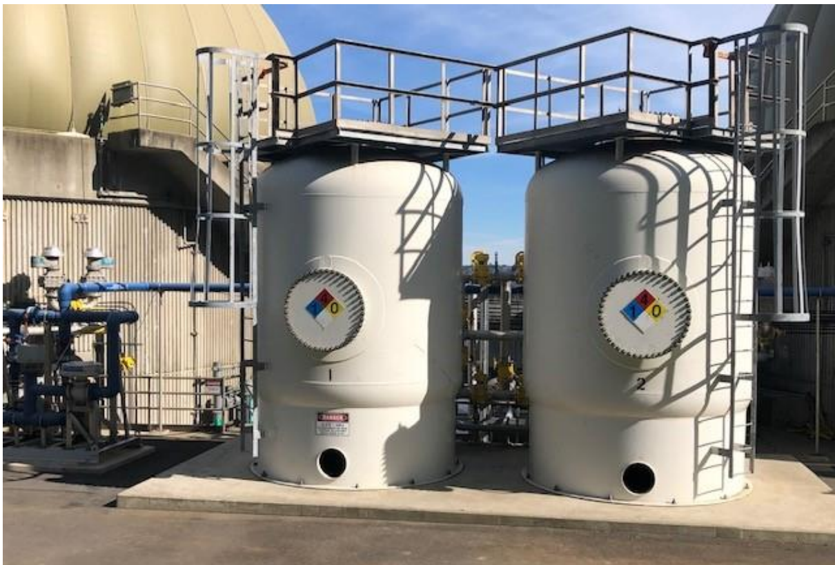
Figure 5. CMSA anaerobic digesters, and hydrogen sulfide media filters that remove hydrogen sulfide from the biogas before it is sent to the cogeneration engine. Source CMSA.
