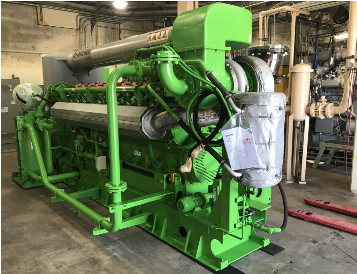
Figure 4. New Jenbacher Cogeneration Engine awaiting installation, with existing engine in background.
