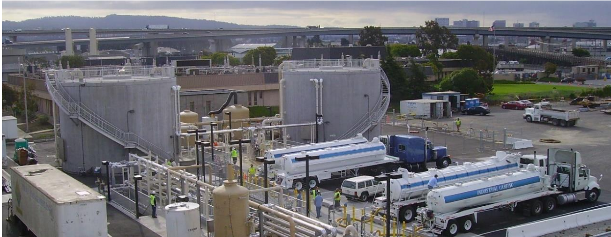
Figure 2. Two above-ground blend tanks at the EBMUD liquid HSOW receiving and blending facility, where food slurry, liquid HSOW, and wastewater treatment streams are blended before entering the digester.
