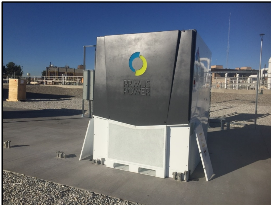
Figure 4-3. A VVWRA flow cell battery.
