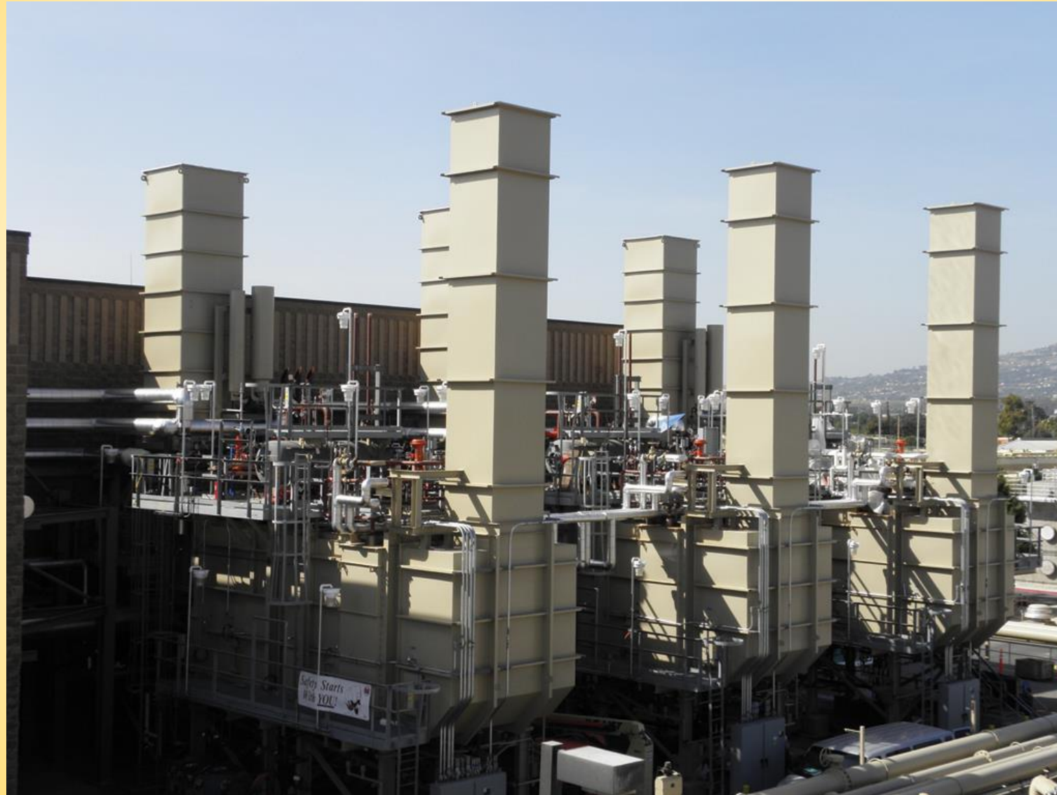
Carlton Joint Water Pollution Control Plant, LA County
