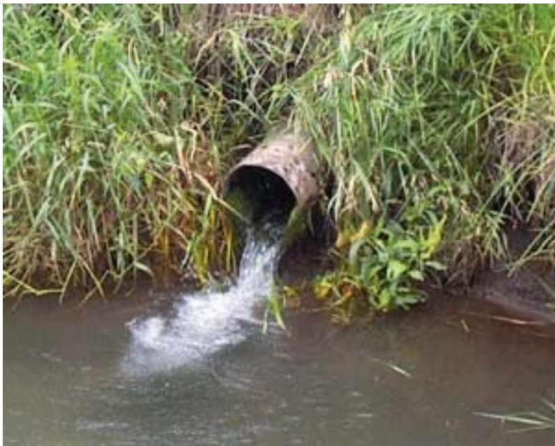
Figure 15. Drain tile outlet discharging to a ditch or stream (Photograph from National Soil Tilth Laboratory, 2004).
