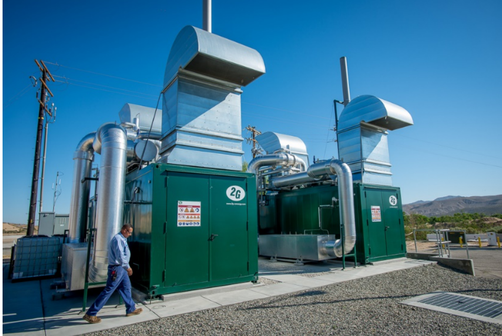
Figure 4-2. VVWRA 2G Generators.
