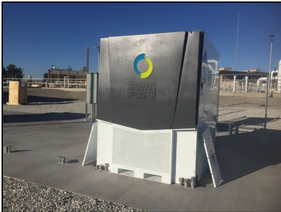
Figure 4-3. A VVWRA flow cell battery.
