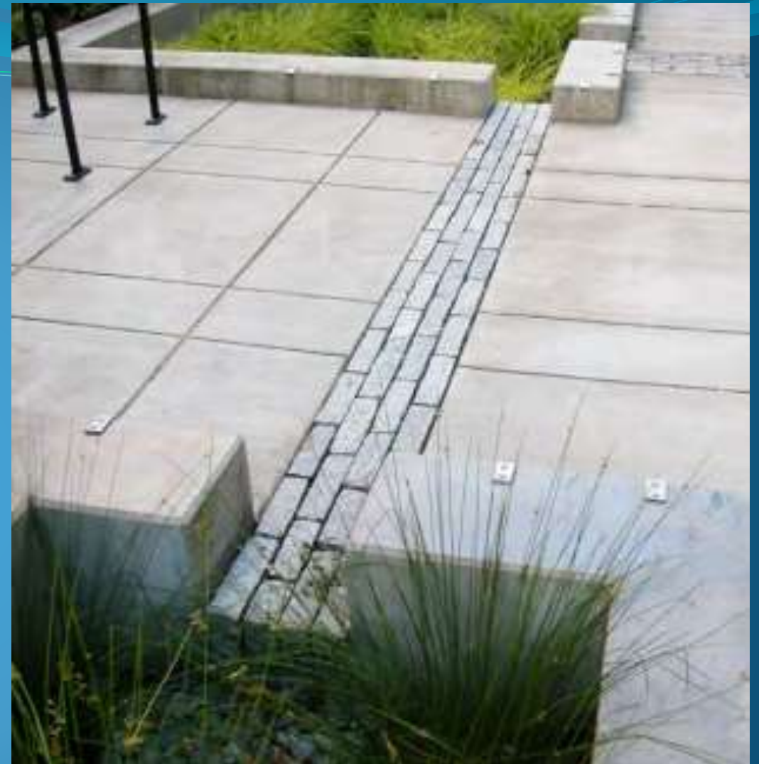
PSU Stephen Epler Hall. Stormwater from the impermeable plaza area is directed to bands of granite stone that are strategically placed at low drainage points to convey stormwater to a series of flow-through planters. Image Source: Low Impact Development Approaches Handbook by Clean Water Services, Portland Oregon.
